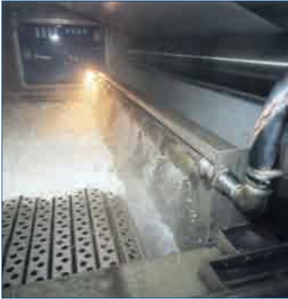
End of the first conveyor
